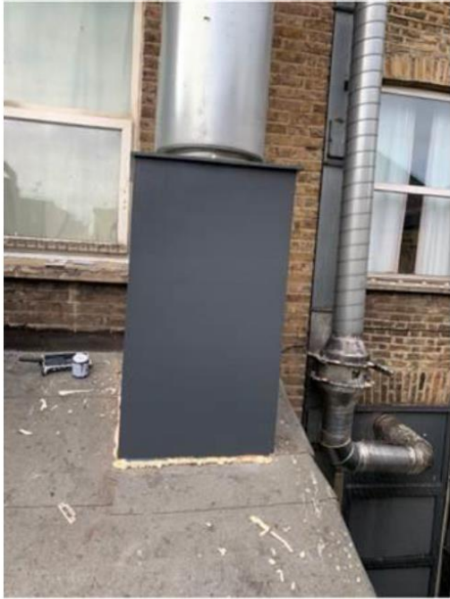
Figure 3: Acoustic enclosure around fan
