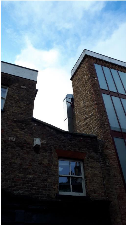
Figure 2: Extract ducting to the rear
